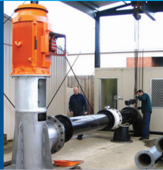
The Pomona Pump test facility
